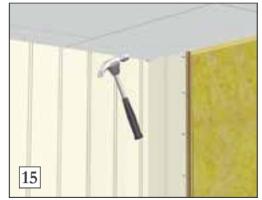
15) The panel is nailed in the nail lip. In the corner, the panel is nailed visibly with dive pins (by hand). Secure top and bottom as usual. Use correction paint (in correct colour) to cover the visible nails.
